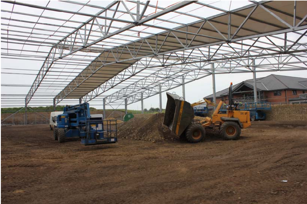
BUILDING WORK: Rubb is constructing the new indoor training facility for SAFC
